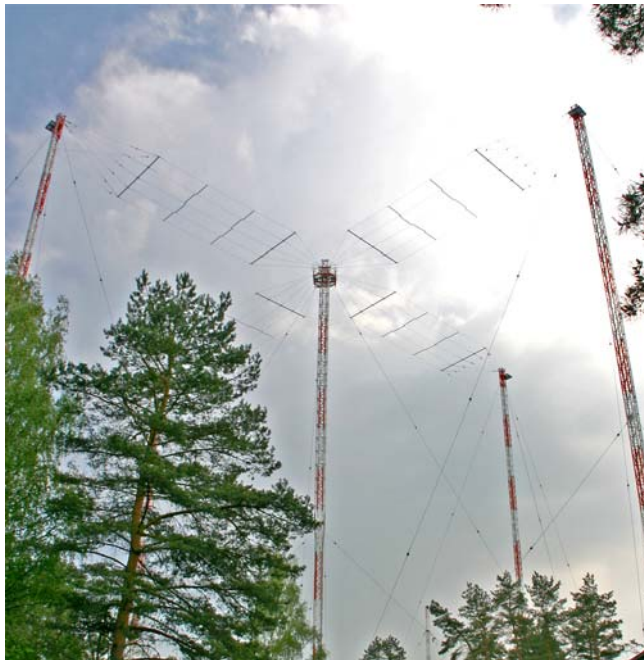
Horizontal cross dipole antenna for MW broadcasting in Mainflingen (Germany)
